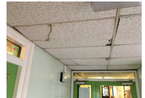
Ceiling tiles- require replacement
