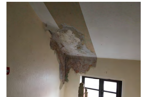
Severe water damage above staircase
