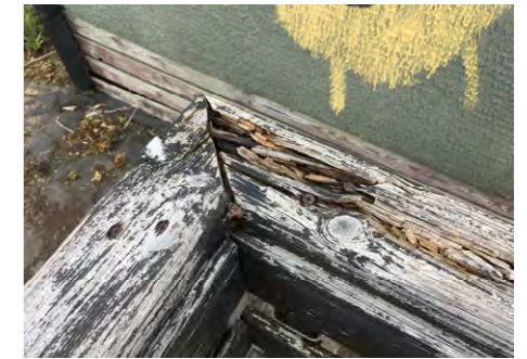
Poor condition of ramp to temporary classroom
