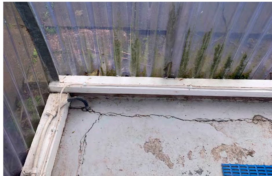
Cracked concrete floor to the swimming pool, with algae growth on the polytunnel roof.
