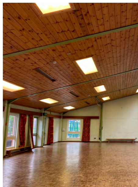
Existing hall ceiling which is subject to leaks and requires remedial works
