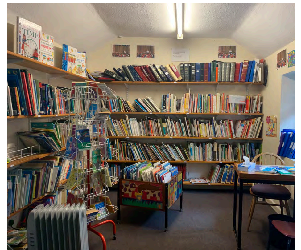
Library space used for 1-to-1 teaching, but suffering from damp.
