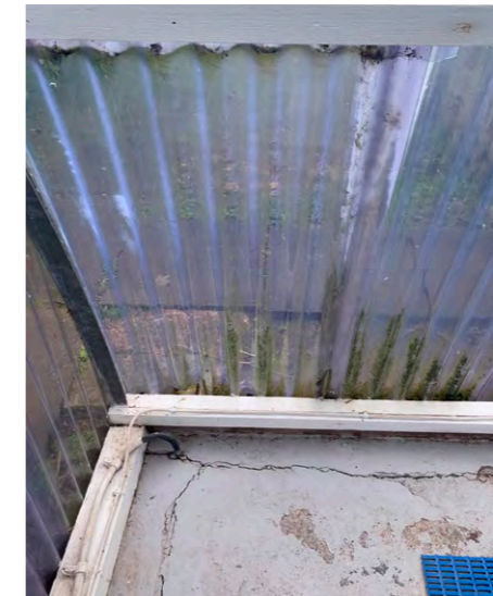
Poor condition swimming pool poly tunnel roof and concrete slab
