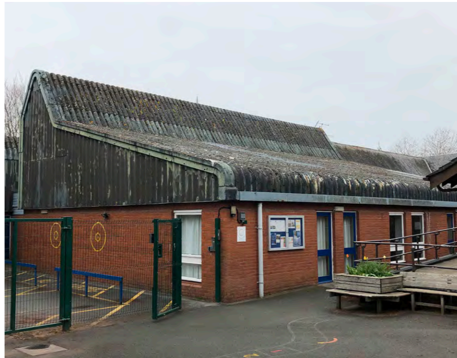
Asbestos cement sheet roof to hall and classrooms to the front of the site
